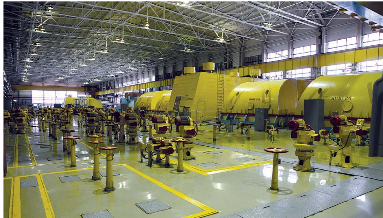
Premises of Leningrad nuclear power-plant
